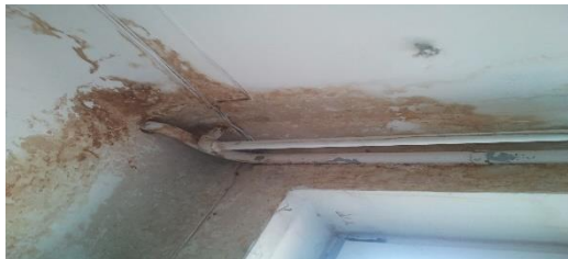
Figure 4 – The microbiological corrosion in industrial building
