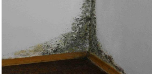
Figure 5 – Biological corrosion in animal farm
