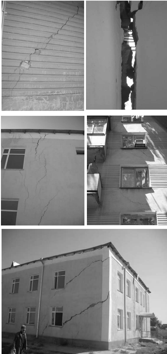
Fig. 1. Damages of buildings bearing walls in seismic areas by substantial differential settlements of soil base
